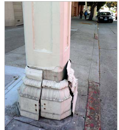
Due to structural failing, the OCS support poles/streetlights along Van Ness Avenue would be replaced under all alternatives, including the No Build Alternative.
