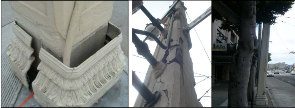
Figure 4.4-5: Damaged and Leaning OCS Support Pole/Streetlights
