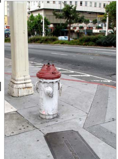
Due to the close proximity to existing facilities, some utilities would require relocation or modification to maintain access for utility providers.
