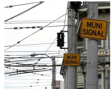
Muni Overhead Contact System (OCS) Photo credit: SFGATE
