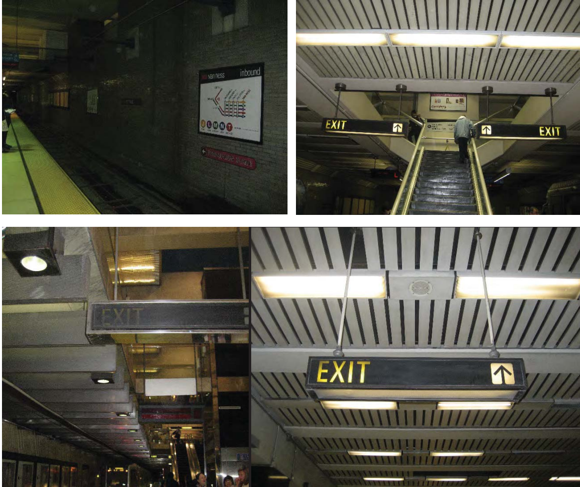
Figure 2: Examples of Low Lighting, Old Fixtures
