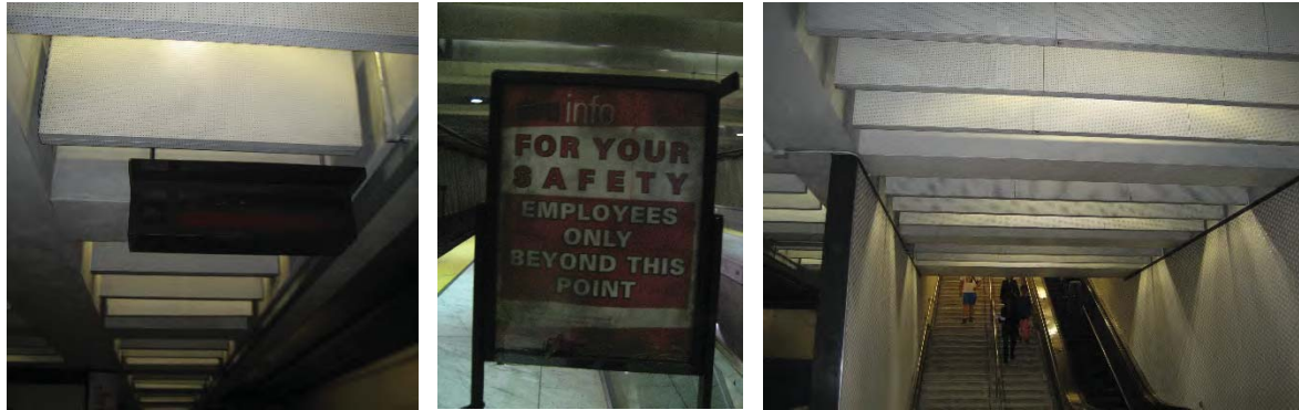
Figure 3: Examples of Acoustic Panels, Lack of Cleanliness
