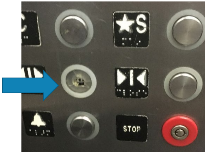
Figure 7. Vandalism to destination buttons at Powell St. Station platform elevator, December 2021.
