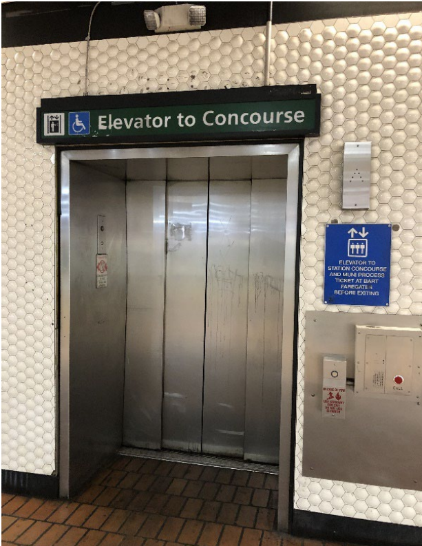
Figure 9. Door vandalism and deterioration of platform elevator at Powell St. Station, December 2021.
