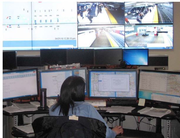
Supported by half-cent sales tax funds, the SFMTA is improving its Central Control and Communications Program.
