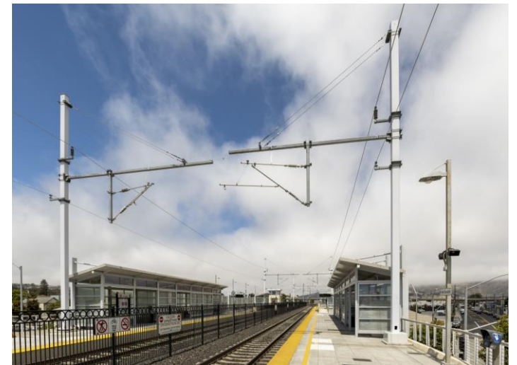
Overhead Catenary System
