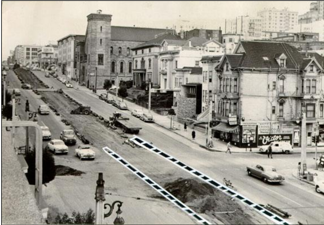
Photograph 27: Track removal on Van Ness Avenue at Vallejo Street in 1952. Note contrasting color of finials and brackets. Also, the result of the WPA street widening (sidewalk narrowing) project is still visible in different color of pavement along sidewalks. Photograph courtesy of San Francisco Public Library Historical Photograph Collection.
