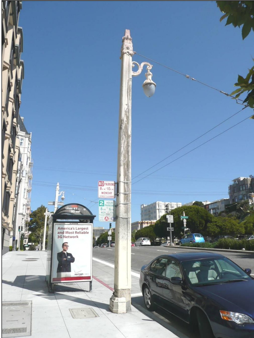
Photograph 4: Part of base missing, Pole 265, between Greenwich Street and Filbert Street, 4/1/2009.
