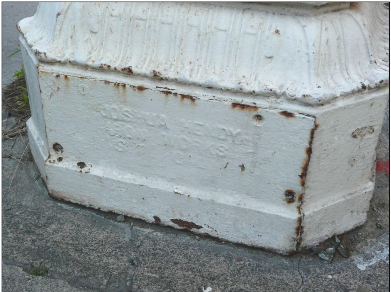
Photograph 7: Mark of "Joshua Hendy Iron Works, S.F., Cal." on original base access door on Pole 298, southeast corner of Van Ness Avenue and Francisco Street, 4/1/2009.
