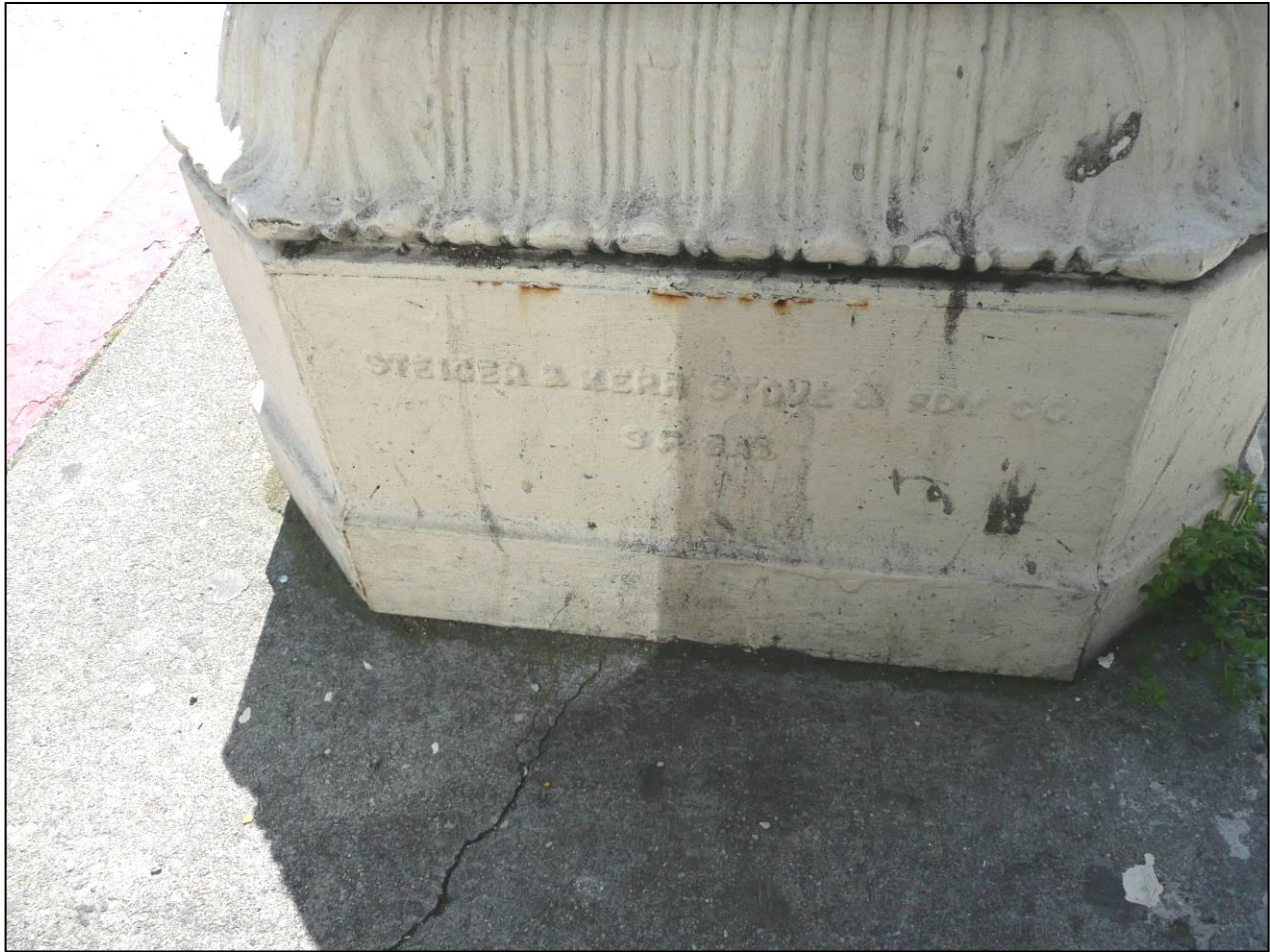
Photograph 8: Mark of “Steiger & Kerr Stove & Foundry Co., SF CA,” on iron replacement base access door on Pole 211, northwest corner of Van Ness Avenue and Pacific Street, 4/1/2009.
