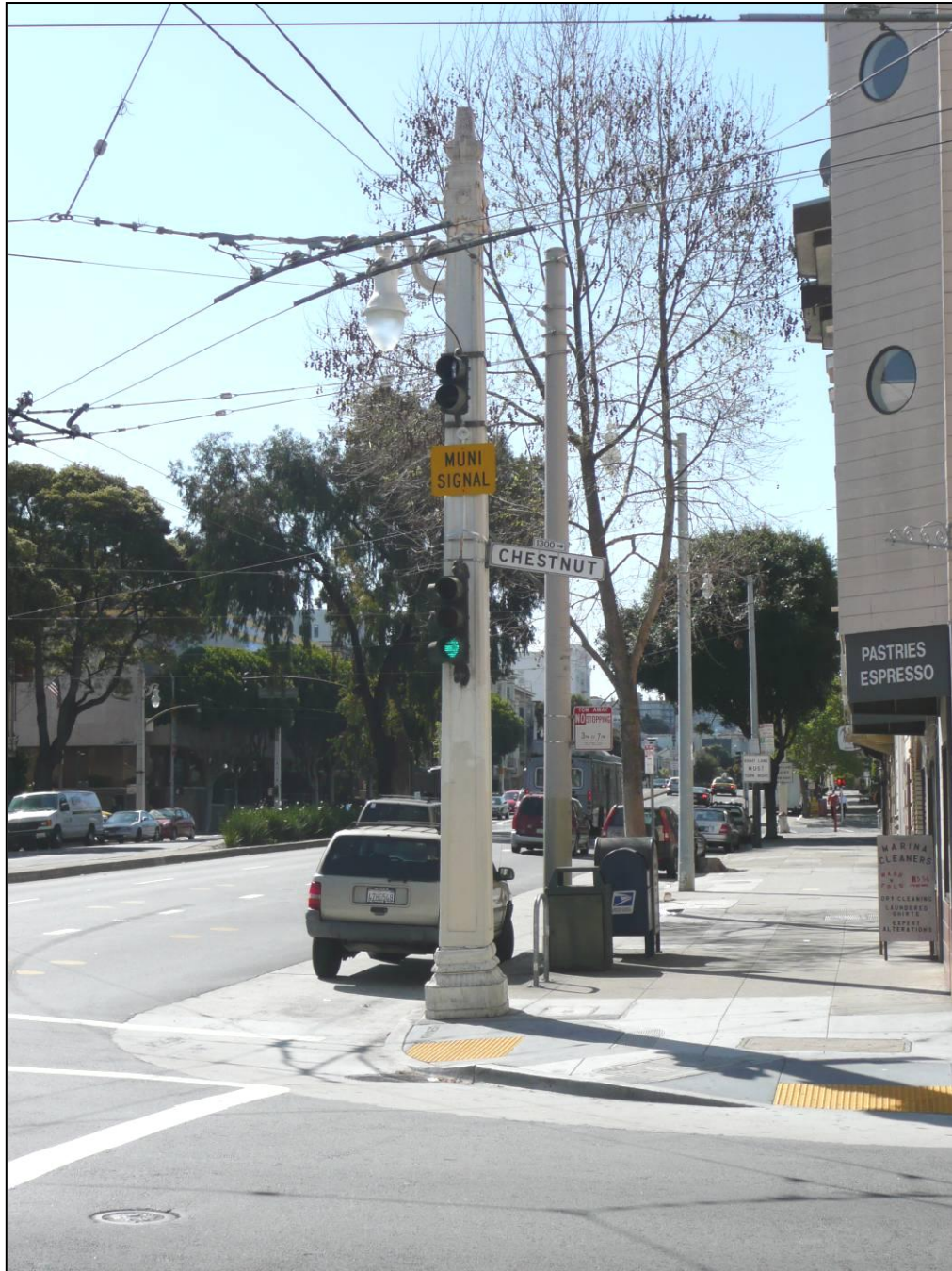
Photograph 5: Electric traffic signal and MUNI signal equipment inserted and signage added to Pole 287, southwest corner of Van Ness Avenue and Chestnut Street, 4/1/2009.
