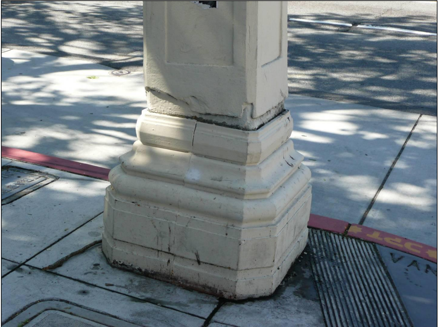
Photograph 9: Replacement fiberglass base without foliated details or access doors, Pole 228, southeast corner of Van Ness Avenue and Vallejo Street, 4/1/2009.
