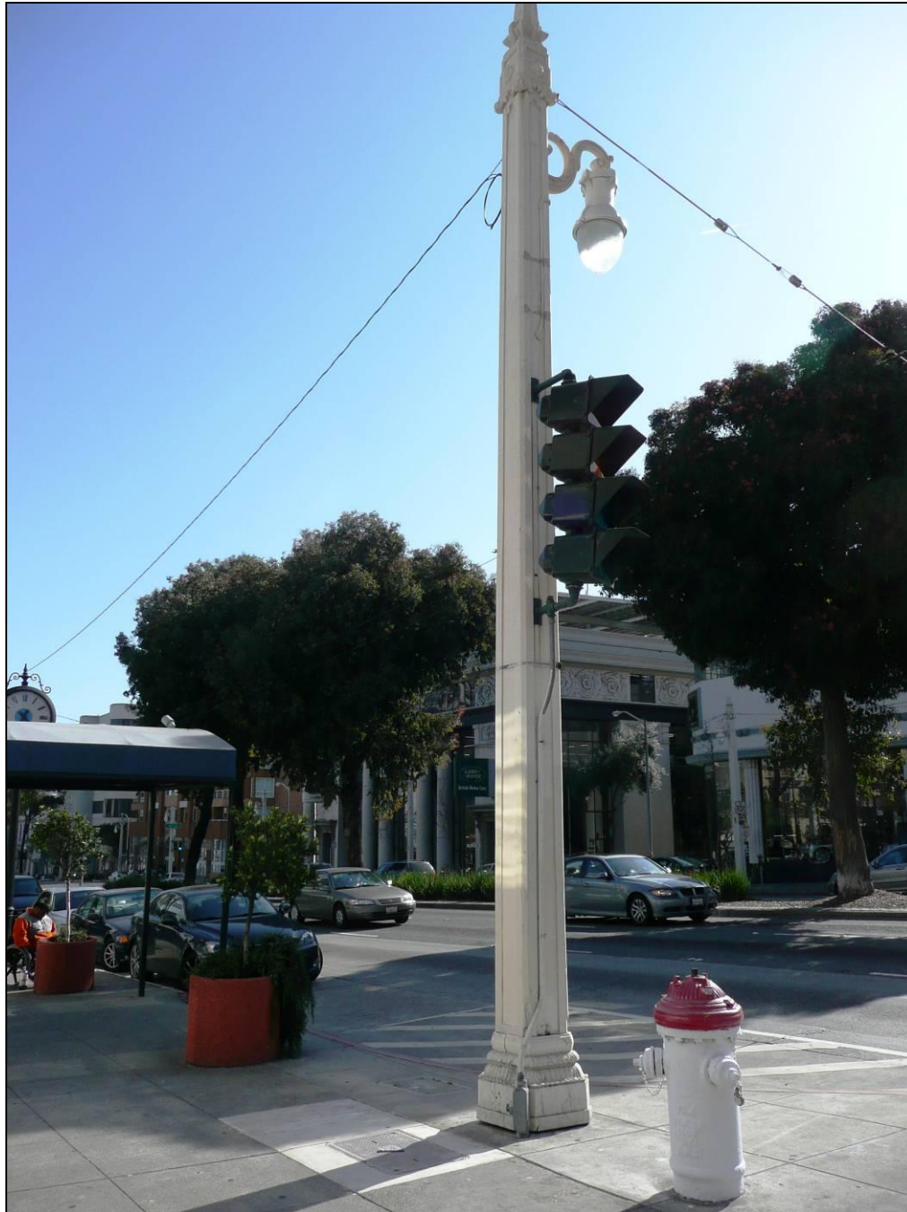
Photograph 22: Traffic signal equipment inserted in Pole 98, Van Ness Avenue and O'Farrell Street, 4/1/2009 (also shown in Photograph 20 above).
