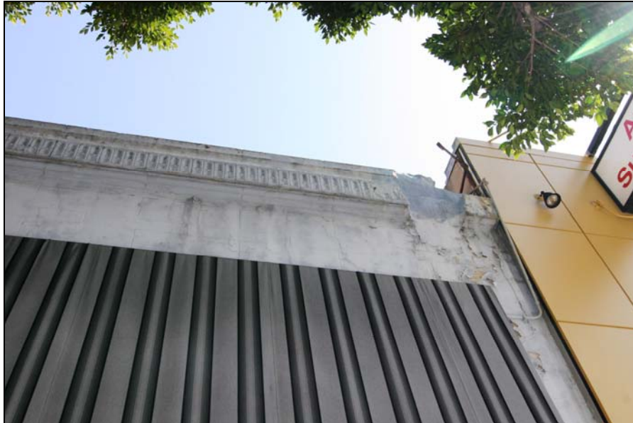
Photograph 2: 1940 Van Ness Avenue, detail of deteriorated façade, camera facing east, 3/8/09
