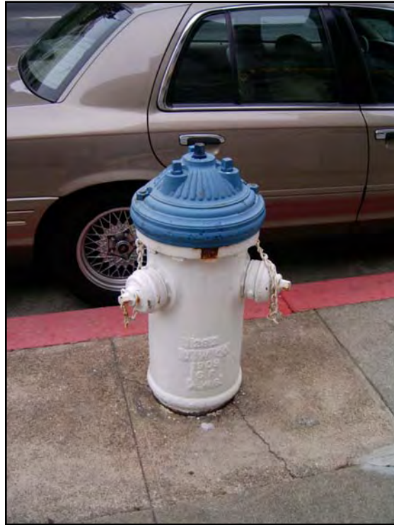
Fire Hydrants, east side of Van Ness Avenue, facing north-west.
