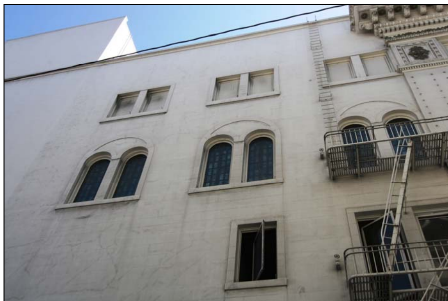
Photograph 5: 1320 Van Ness Avenue, stained glass windows on secondary elevation, camera facing south, 3/8/09
