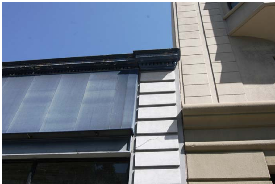
Photograph 2: 1730 Van Ness Avenue, detail of restuccod façade, aluminum screen and original cornice, camera facing east, 3/8/09
