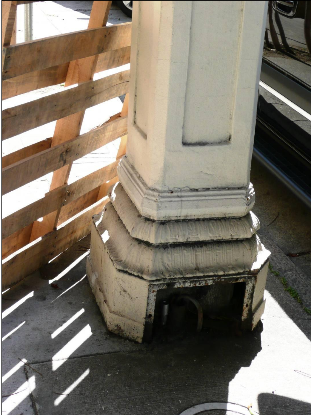
Photograph 3: Original pole and base, missing access door, Pole 196, east side of Van Ness between Jackson and Washington, 4/1/2009.
