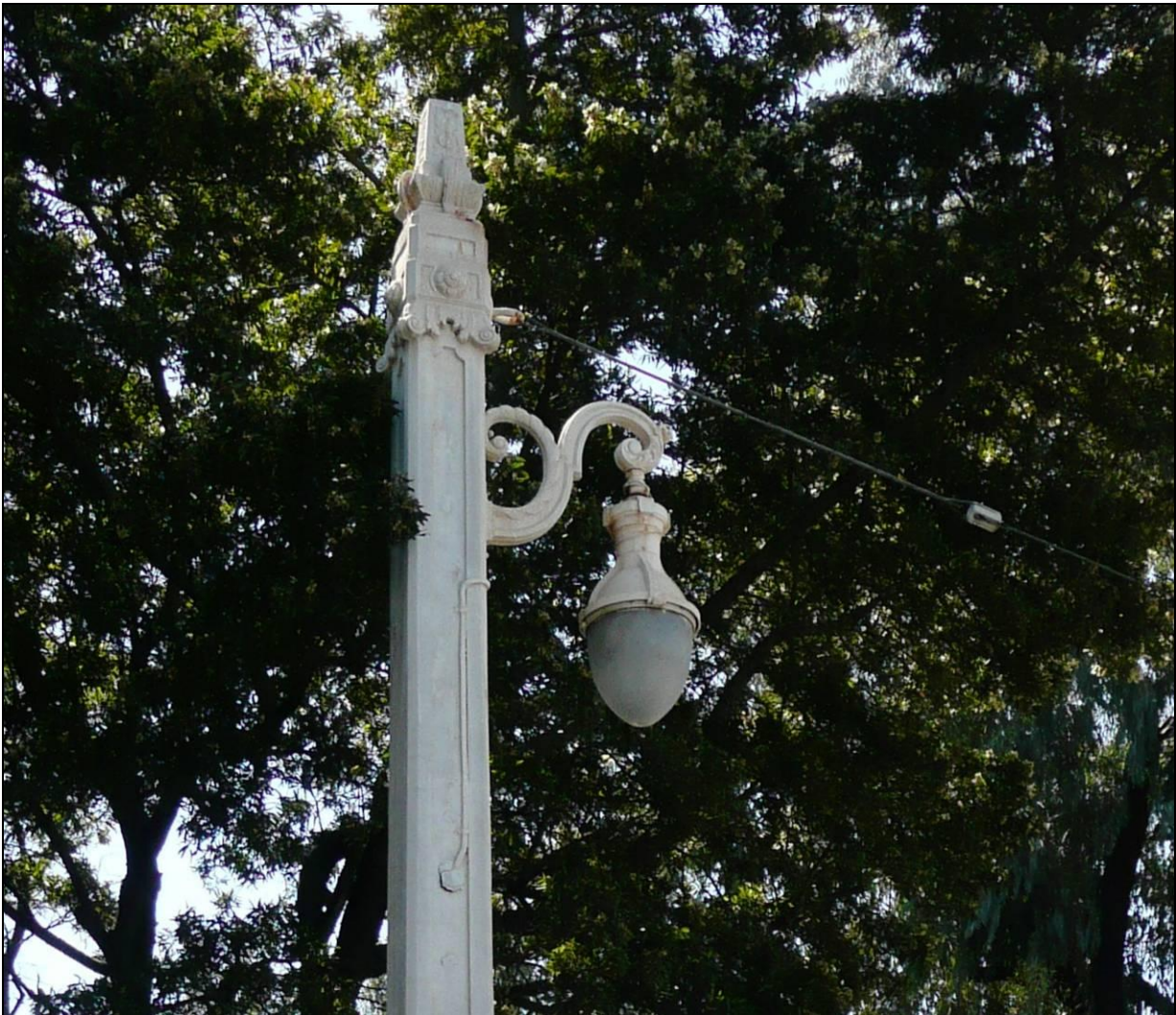
Photograph 10: Detail showing exterior wiring inserted in Pole 264, with original finial and 1936 bracket and modern luminaire, Van Ness Avenue between Greenwich and Filbert streets, 4/1/2009.
