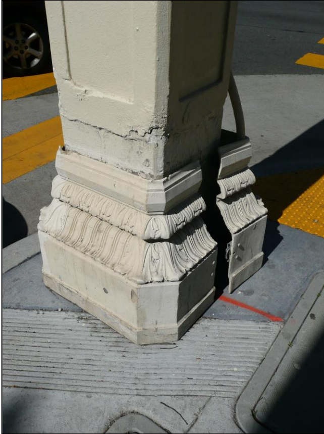
Photograph 15a and 15b: Example of fiberglass replacement base (this one with foliated detailing), no access doors, Pole 308, at the southeast corner of Van Ness and Bay, 4/1/2009.
