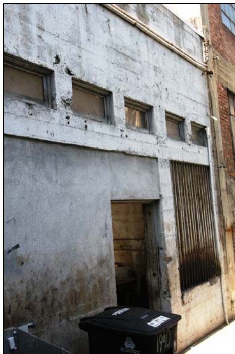
Photograph 3: 1940 Van Ness Avenue, rear of building with filled in garage door, camera facing northwest, 3/8/09
