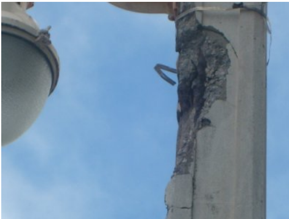
Figure 2.4: Exposed Rebar, Hayes and Van Ness Avenue (Pole 18)
