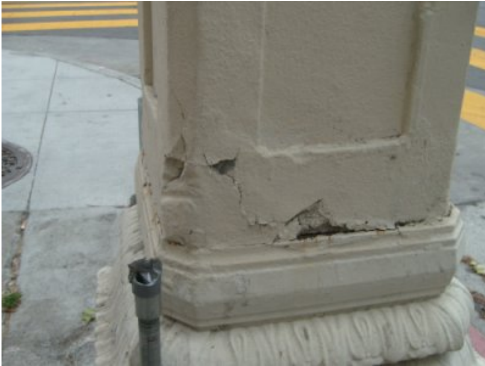
Figure 2.5: Cracked Base, Francisco and Van Ness Avenue (Pole 297)
