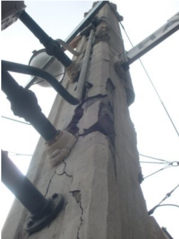
Figure 2.3: Concrete Spall, Hayes and Van Ness Avenue (Pole 17)
