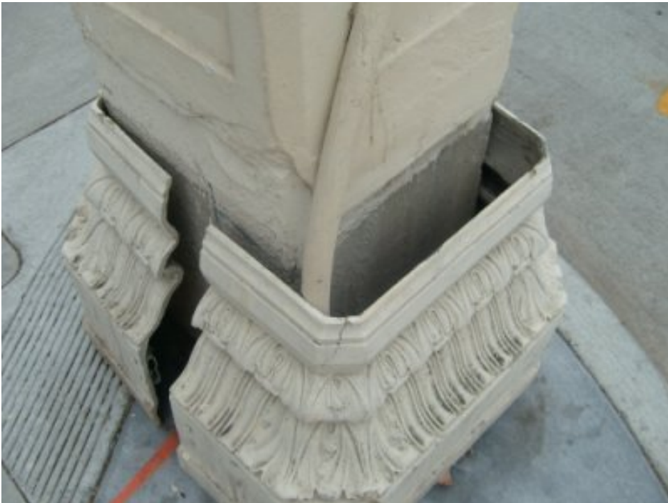
Figure 2.6: Detached Fiberglass Replacement, Bay and Van Ness Avenue (Pole 308)
