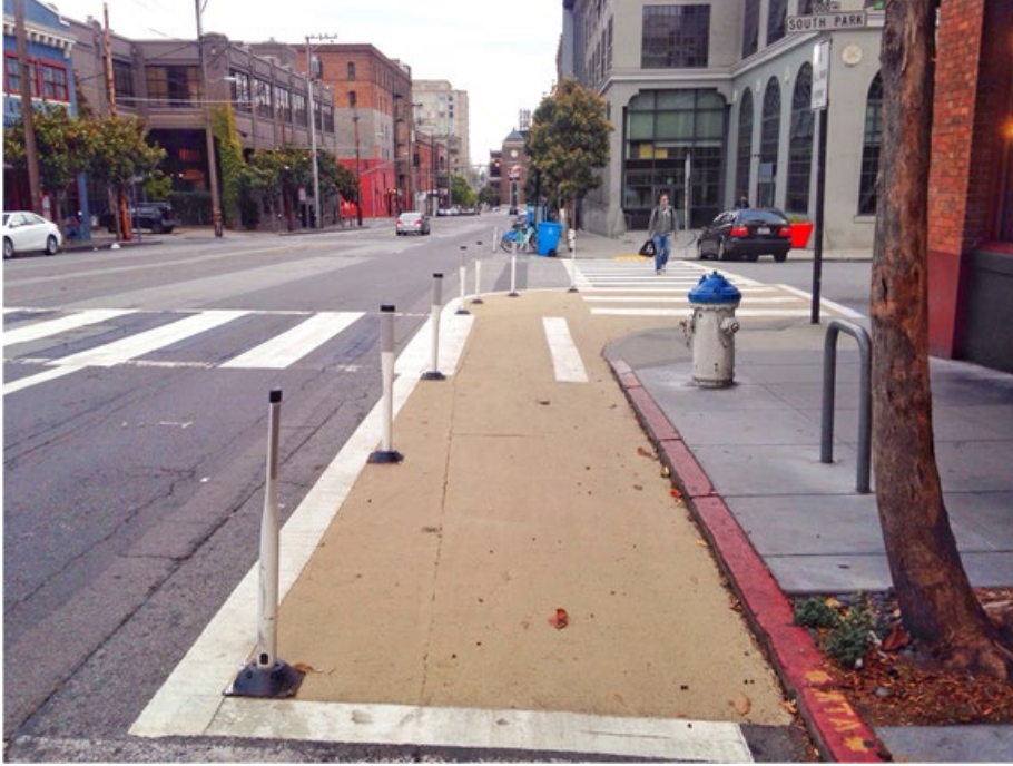
Typical Before – Painted Safety Zone
