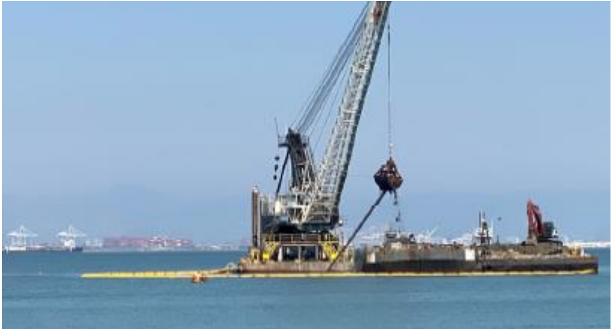
Figure 7: Dredge using 6 cy bucket to remove full pile from MBFL dredge area prior to NUAD dredging, Sept 4, 2020.
