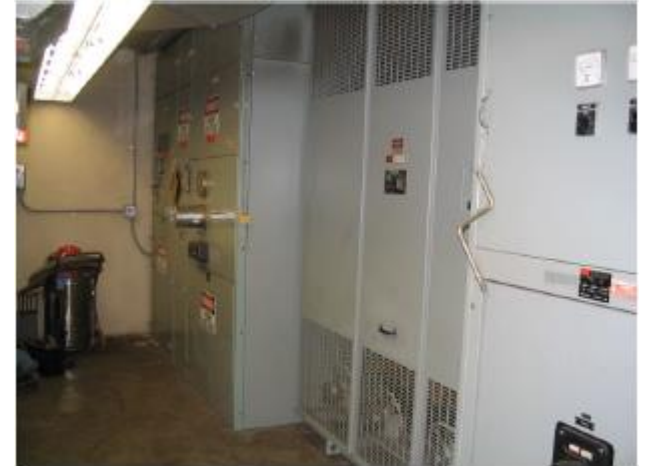
Medium Voltage Service Entrance Switchgear, 2.5 MW Medium Voltage Transformer and 480 V Switchboard
