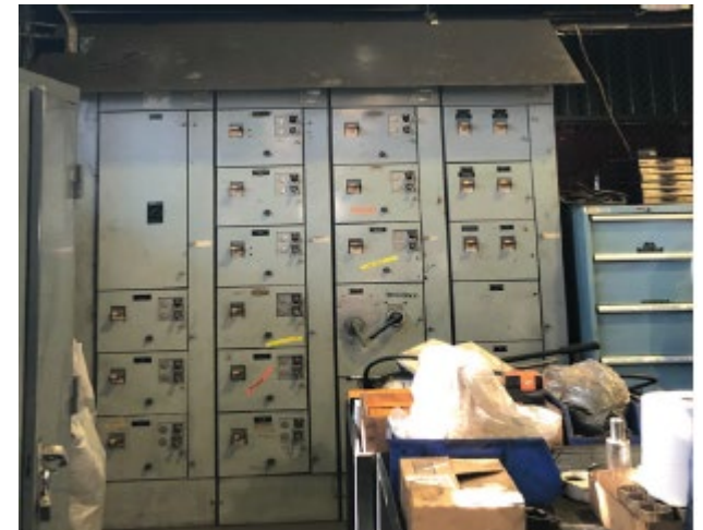
Motor Control Center (MCC)
