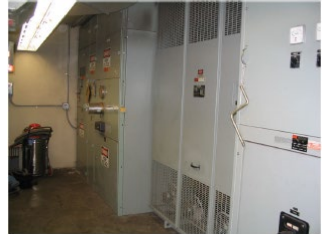
Medium Voltage Service Entrance Switchgear, 2.5 MW Medium Voltage Transformer and 480 V Switchboard
