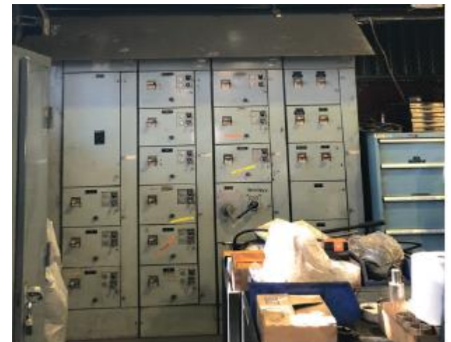
Motor Control Center (MCC)
