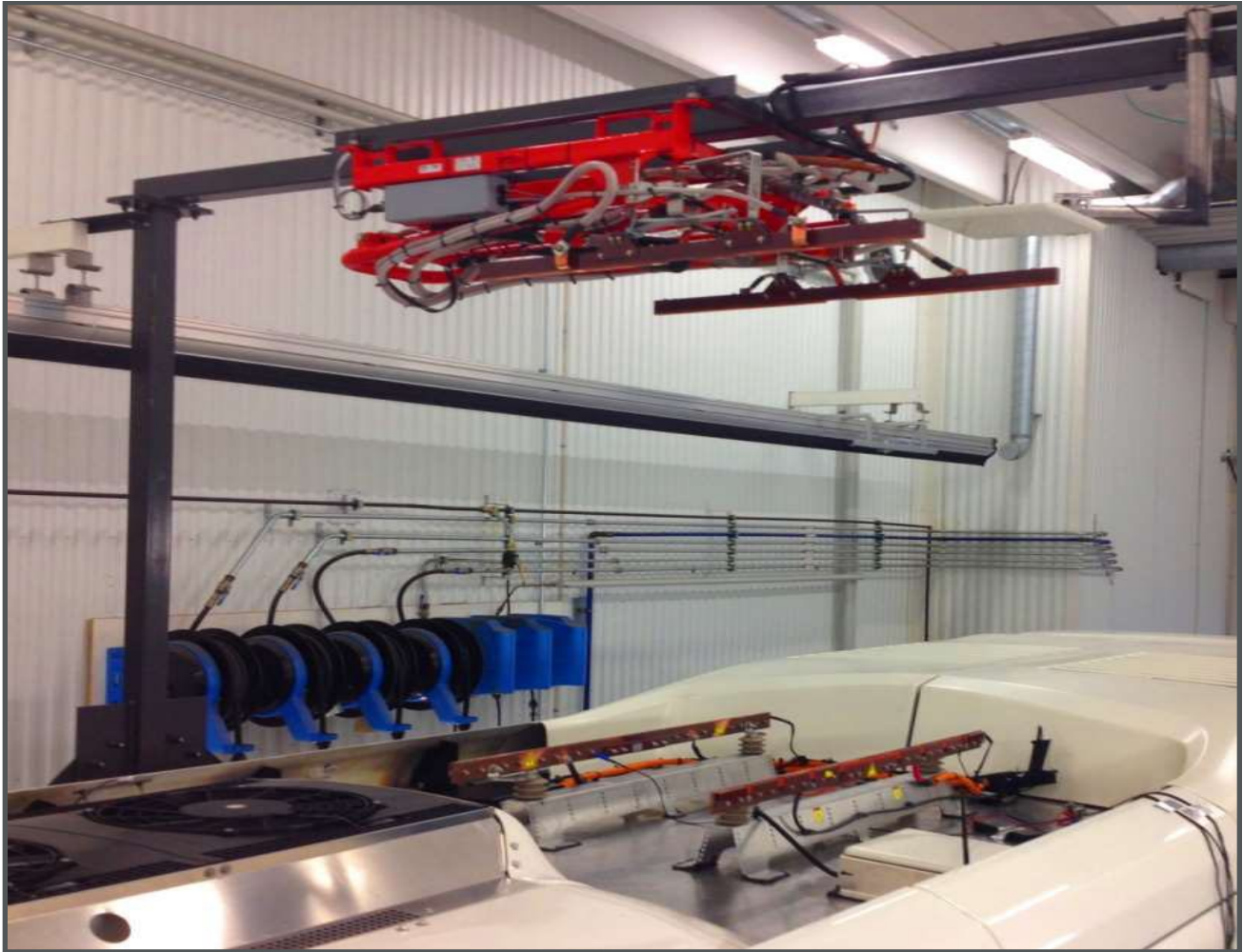
Figure 3-1. Inverted Pantograph and Charge Rails
