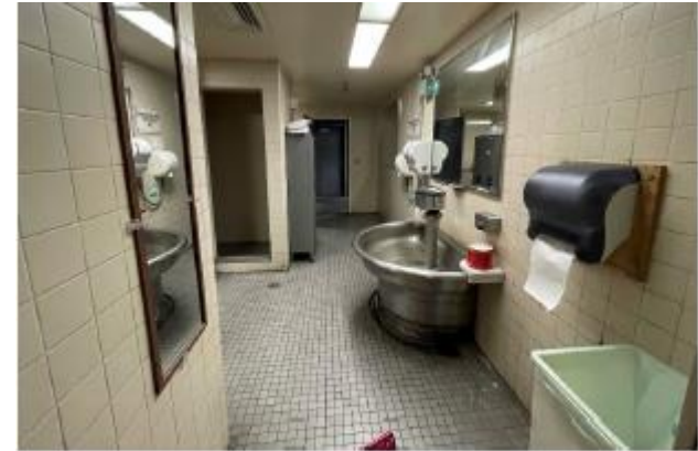
Non-compliant lavatory and shower (Men 203).
