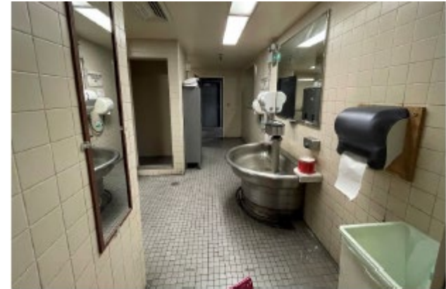
Non-compliant lavatory and shower (Men 203).
