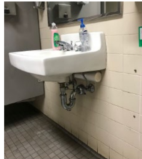
Non-compliant lavatory (Women 106).
