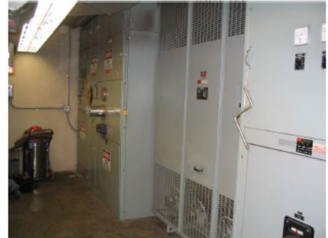
Medium Voltage Service Entrance Switchgear, 2.5 MW Medium Voltage Transformer and 480 V Switchboard
