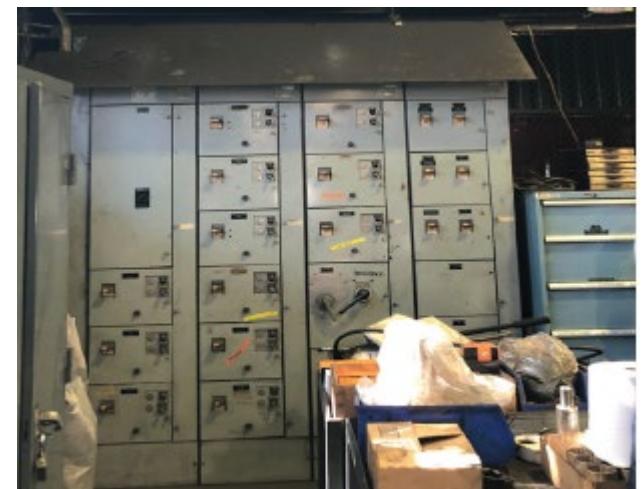
Motor Control Center (MCC)
