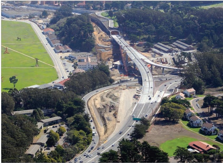
Construction of the Southbound Battery Tunnel and Presidio Viaduct were completed as part of Presidio Parkway Phase I.
