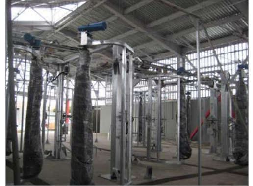
Phase I of the Islais Creek Maintenance facility project includes a state-of-the-art vehicle wash system.
