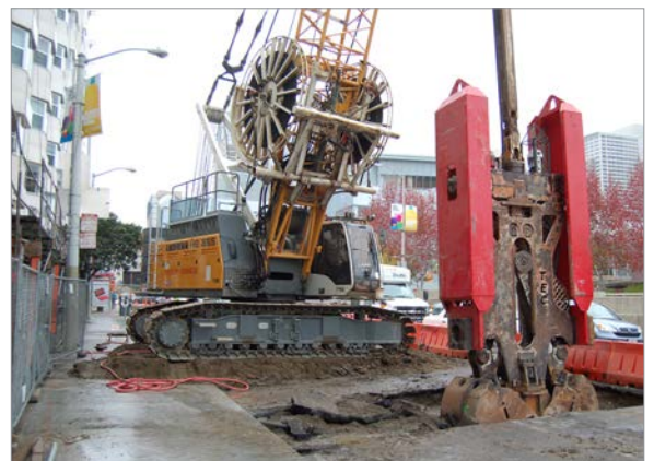
(Top) The cutterhead for "Mom Chung," the first of two tunnel boring machines, being lowered into the 4th Street launch box for assembly. (Bottom) Excavation for the headwalls of the Yerba Buena/Moscone station.
