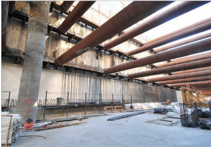
Excavation of the four-block Transbay Transit Center site will be completed in early 2014.
