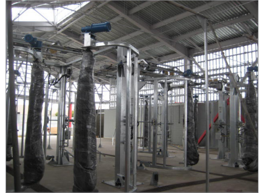
Phase I of the Islais Creek Maintenance facility project includes a state-of-the-art vehicle wash system.
