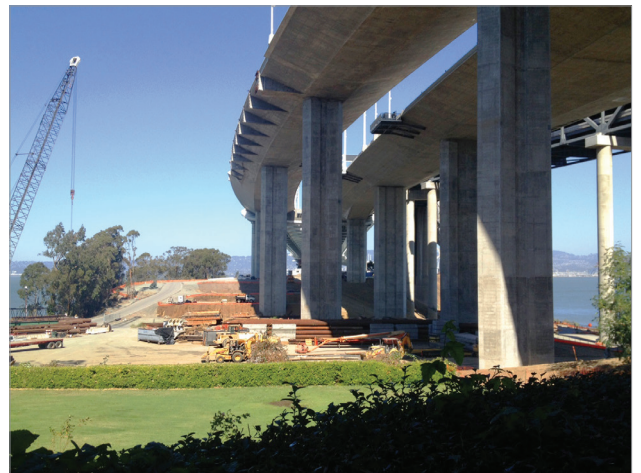
New westbound on and off ramps (on the east side of Yerba Buena Island) will improve access to and from the new Eastern Span of the Bay Bridge.
