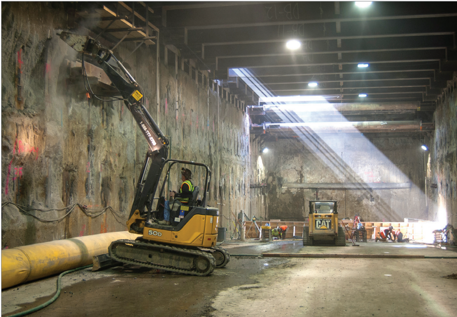
State STIP funds are part of a complex funding plan for the SFMTA’s $1.58 billion Central Subway project. Shown above: constructing the 4th Street launch box for the tunnel boring machines.
