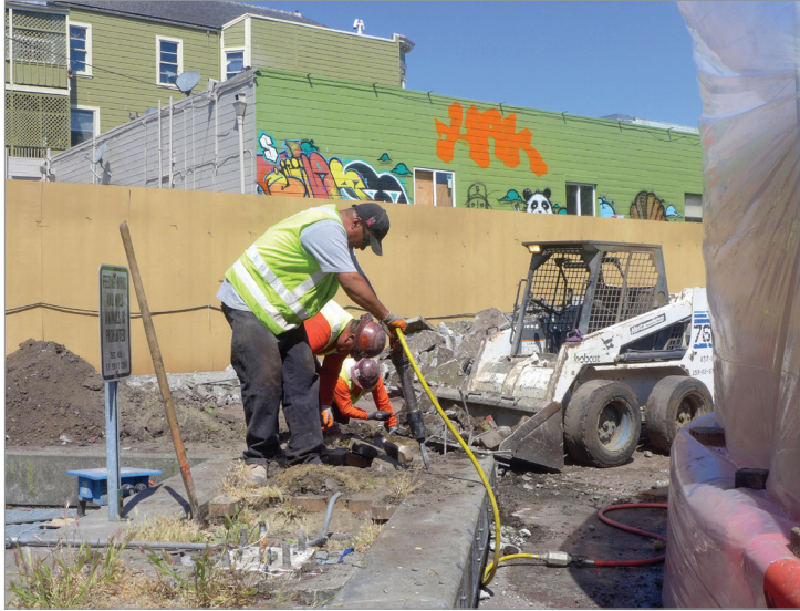
Renovation of the 24th Street Mission BART Station plaza was one of the first projects funded by Prop AA.
