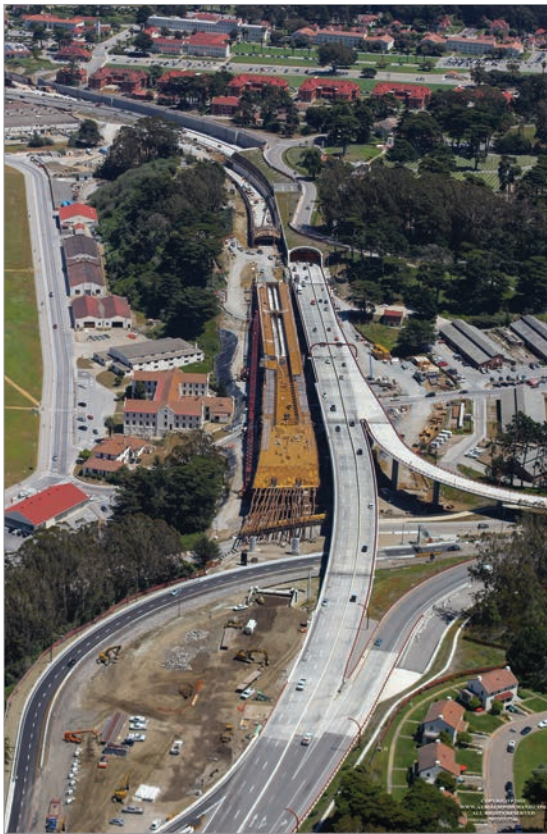
The completion of the southbound tunnels and viaducts will allow for the traffic switch in early summer of 2015.
