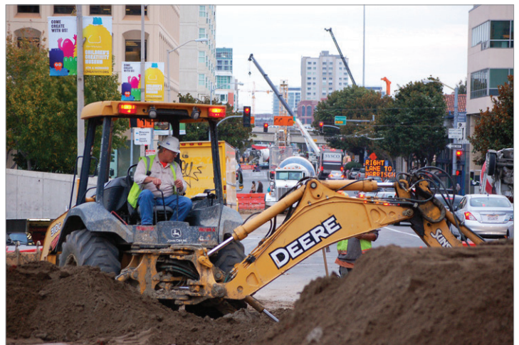
State STIP funds are part of a complex funding plan for the SFMTA’s $1.58 billion Central Subway project. Shown here, excavation for the 4th Street Moscone Center station.
