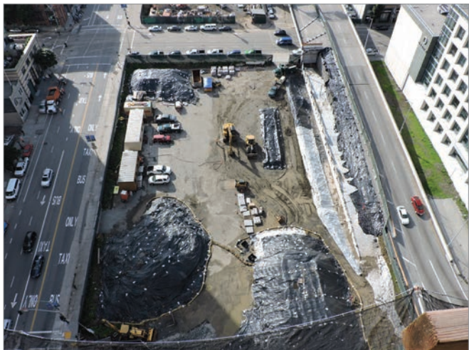
The Folsom Street Off-Ramp Realignment Project has demolished the curved Folsom Street leg of the off-ramp and will reconstruct the ramp to enhance pedestrian accessibility on Fremont Street and provide an enlarged parcel for redevelopment uses.
