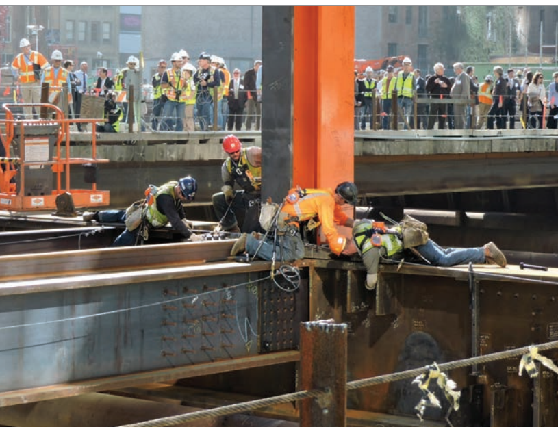
Installation of the first above-ground steel member signaled the start of the above-ground construction phase of the building.
