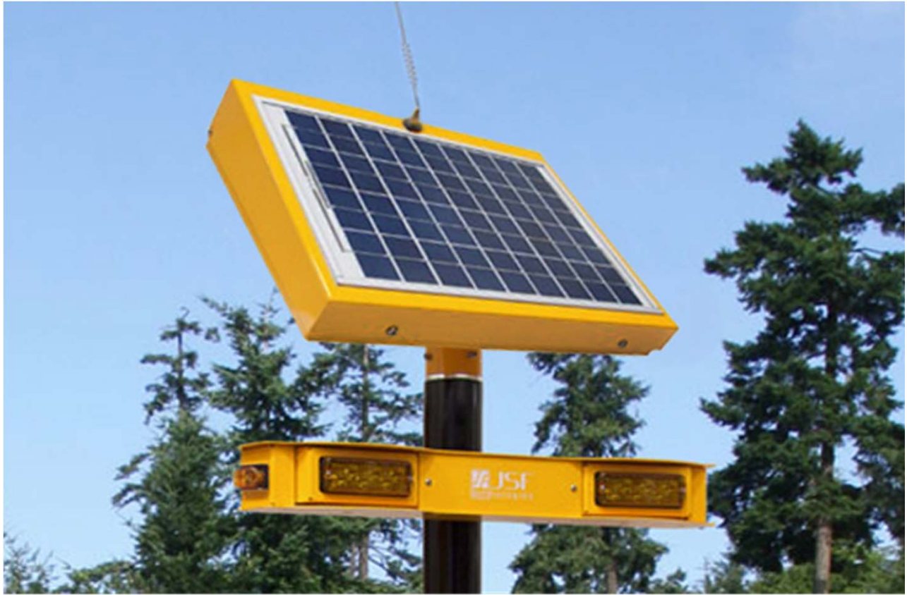
Rectangular Rapid Flashing Beacon and Solar Panel
