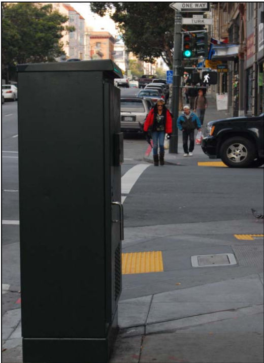
Traffic Controller and new curb ramps
