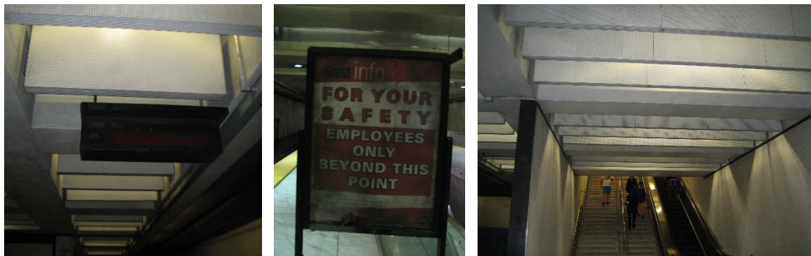
Figure 3: Examples of Acoustic Panels, Lack of Cleanliness
