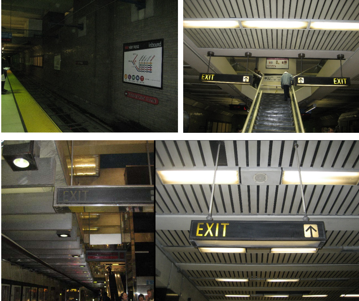
Figure 2: Examples of Low Lighting, Old Fixtures
