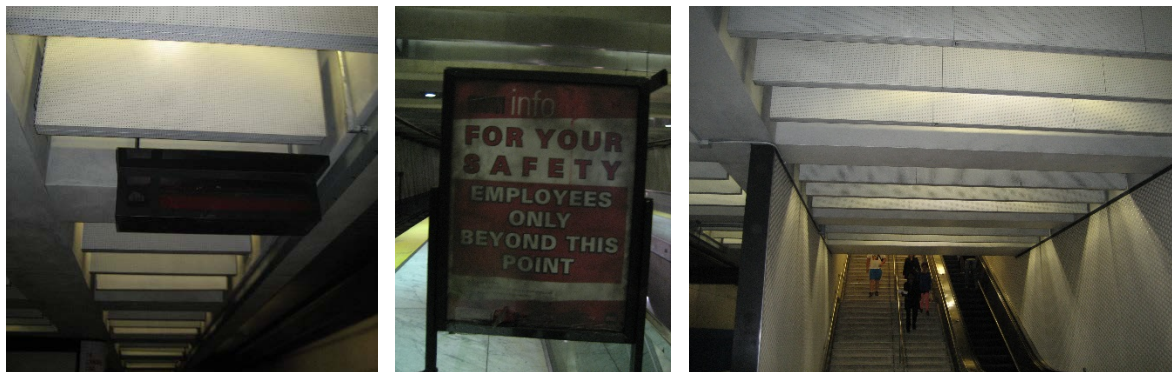
Figure 3: Examples of Acoustic Panels, Lack of Cleanliness
