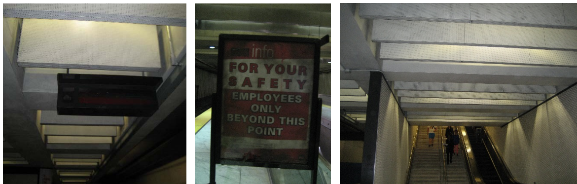
Figure 3: Examples of Acoustic Panels, Lack of Cleanliness
