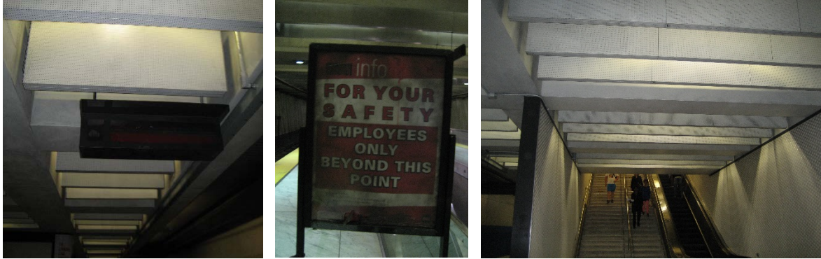
Figure 3: Examples of Acoustic Panels, Lack of Cleanliness
