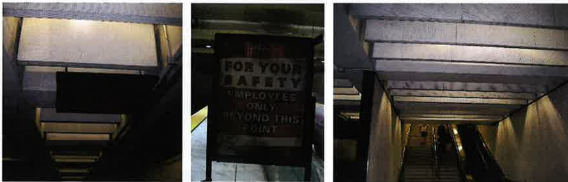
Figure 3: Examples of Acoustic Panels, Lack of Cleanliness
