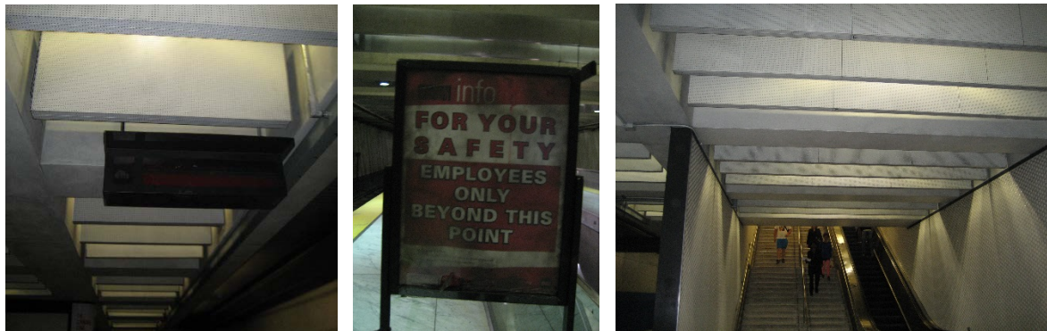
Figure 3: Examples of Acoustic Panels, Lack of Cleanliness
