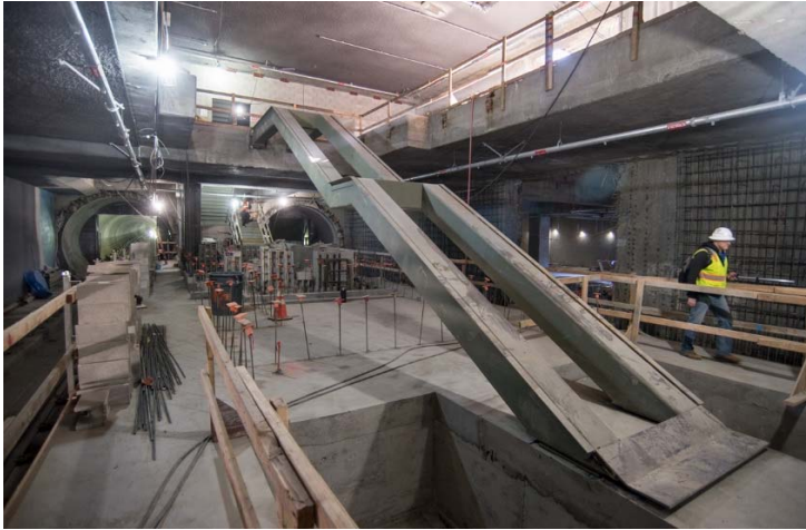
Yerba Buena/Moscone Station: Steel framing for stairs and escalator components are being installed inside the station box under 4th Street.
