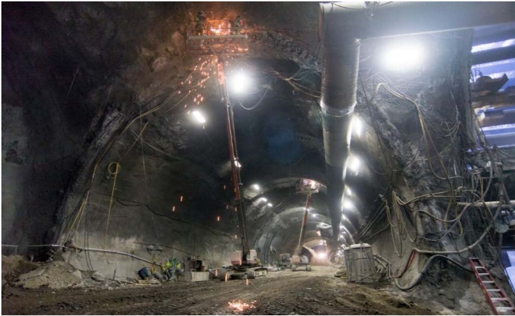
Chinatown Station: The arched station cavern and crossover cavern under Stockton Street are nearly fully excavated.
