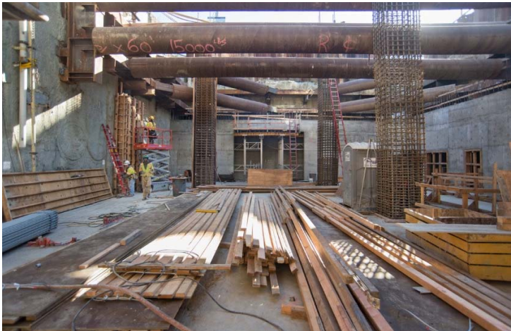
Yerba Buena/Moscone Station: Interior walls and the Mezzanine-level floor slab are being constructed inside the station headhouse.
