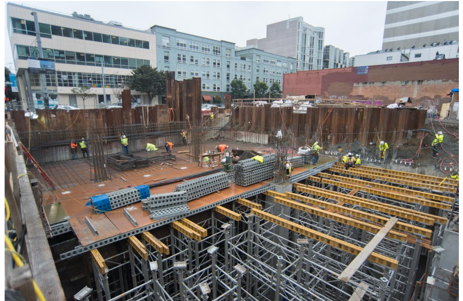
Various stages of roof deck construction can be seen inside the Yerba Buena/Moscone Station headhouse
