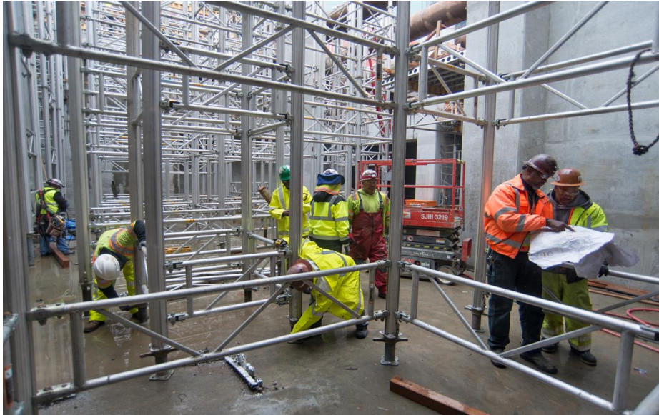
Large sections of scaffolding are being positioned inside the station headhouse to hold up future roof deck concrete forms
