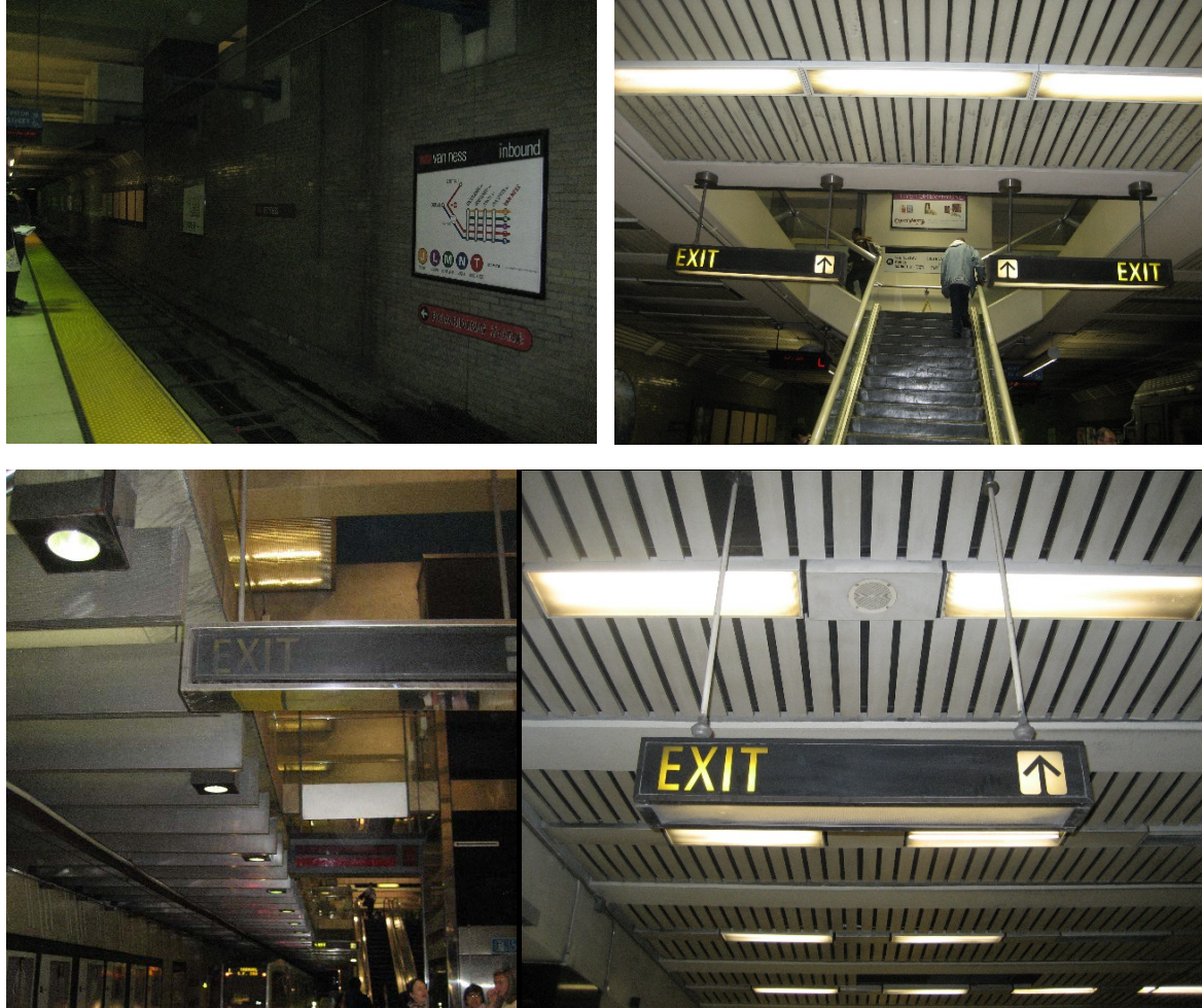
Figure 2: Examples of Low Lighting, Old Fixtures
