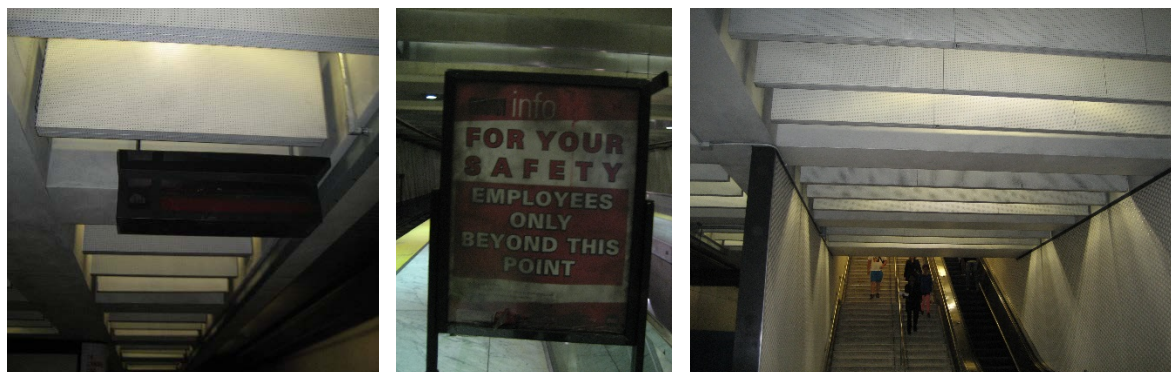
Figure 3: Examples of Acoustic Panels, Lack of Cleanliness
