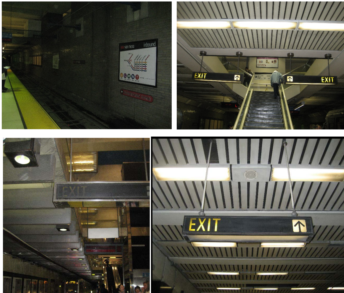
Figure 2: Examples of Lighting Levels and Existing Fixtures
