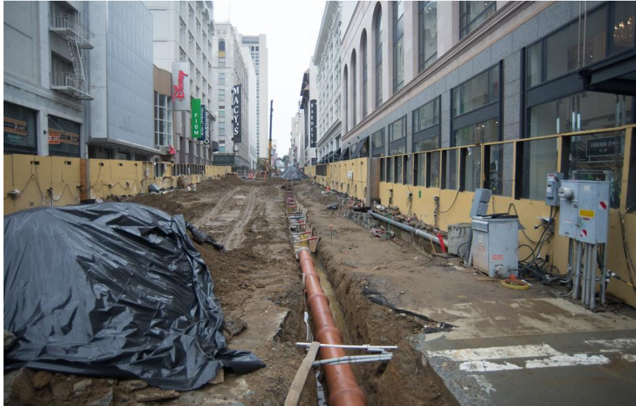
Sewer pipes and other utilities are being installed above the buried roof deck of the Union Square/Market St. Station's south concourse
