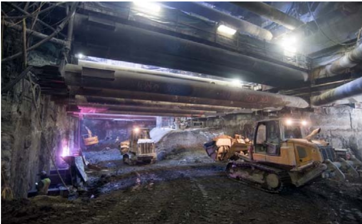
Chinatown Station: Bulldozers line up to offload material during excavation of the station cavern and headhouse.
