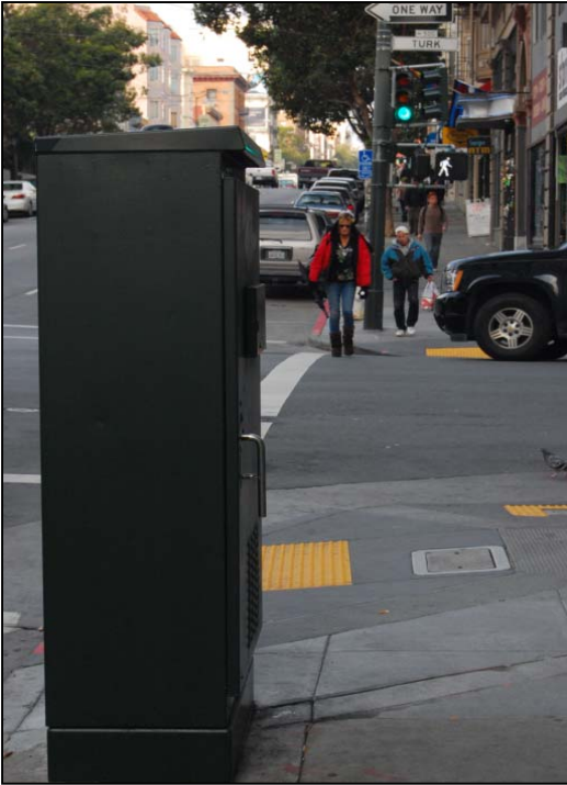
Traffic Controller and new curb ramps
