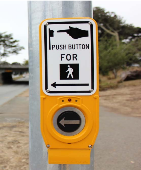
Accessible Pedestrian Signals
