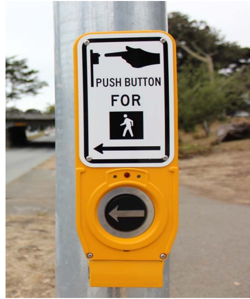
Accessible Pedestrian Signals
