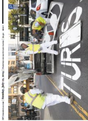
Above: Metropolitan Transportation Agency workers paint dividers for drivers on South Street. Below: Lane along the curb was 'highlighter' at sixth and Howard as part of the Vision Zero walk.
